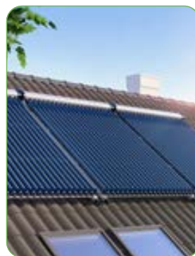
Solar Thermal Panels
