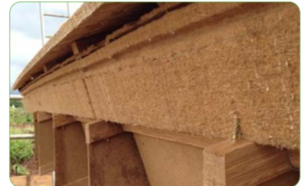
Wood Fibre insulation in timber frame building (source: www.carpenteroak.com )
