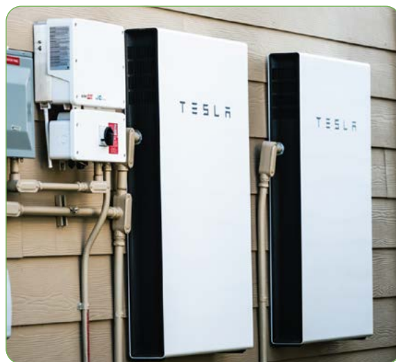
Tesla Powerwall battery system (source: www.ecoaffect.org )
