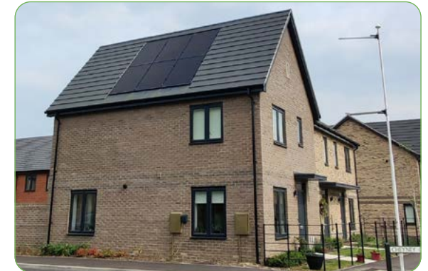
PV panels fitted flush with the roof tiles, Alconbury Weald
